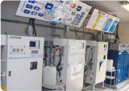
Automatic Wastewater Analyzer
