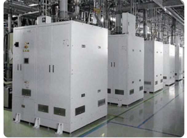
PFCs Abatement Equipment
